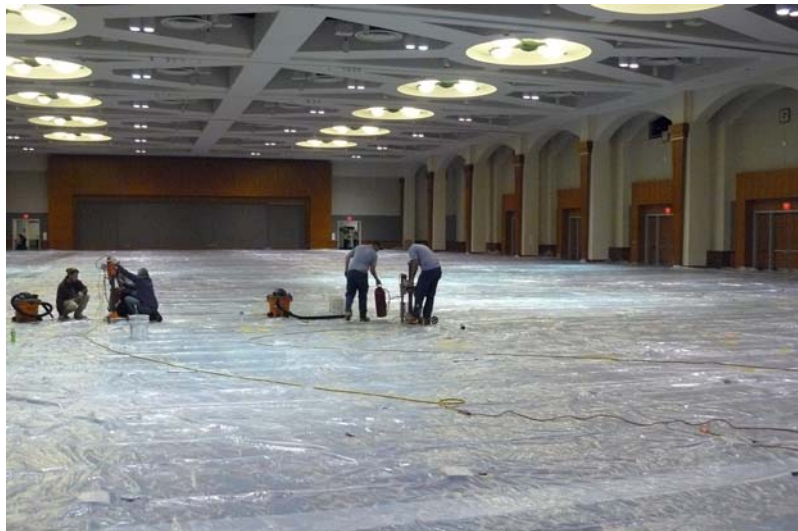
Above: CRC crews work to core drill strategically-placed grouting injection holes within the main ballroom areas of the Frontier Airlines Center. Plastic sheeting appears over the carpeted ballroom floor. Flaps were cut in the carpet for grout injection holes.
