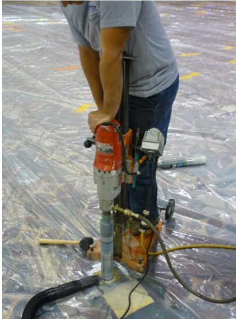
Above: CRC crews core drill strategically-placed grouting injection holes within the main ballroom areas.
