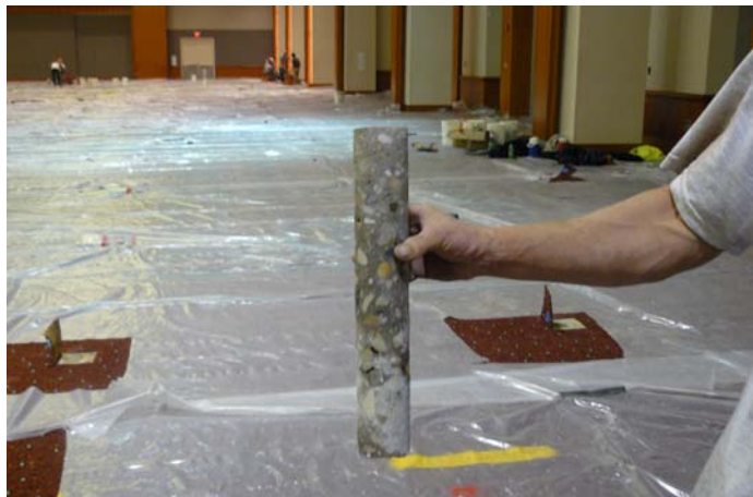
Above: A 14-inch core taken from the interior floor of the Frontier Airlines Center.
